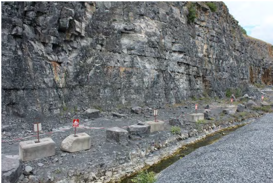
Figure 26 Beneath high face showing rockfalls.
