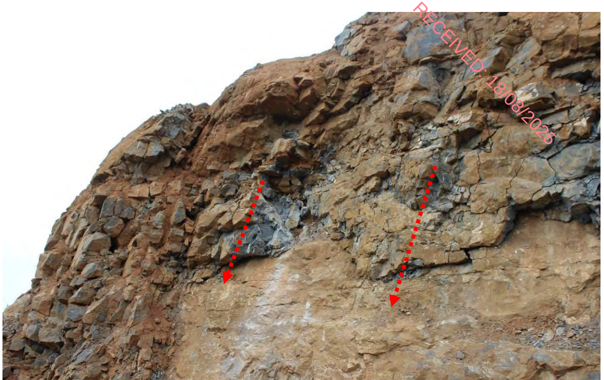
Figure 23 Loose Material in Eastern upper face as evidenced from previous assessment
