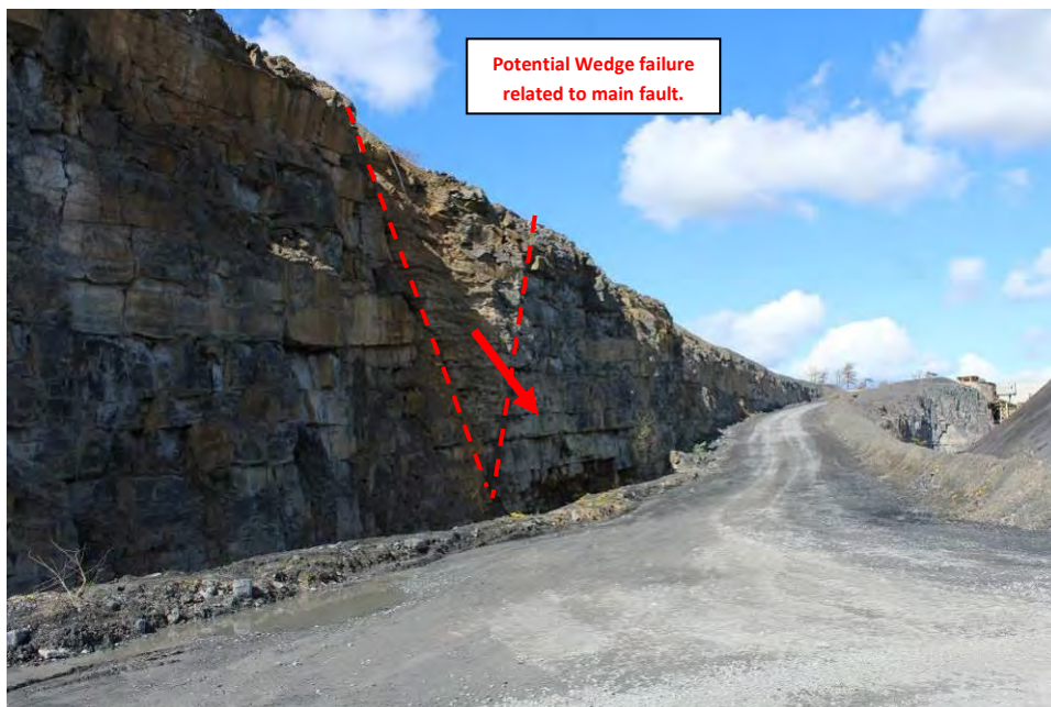
Figure 28 Potential Wedge failure related to main fault
