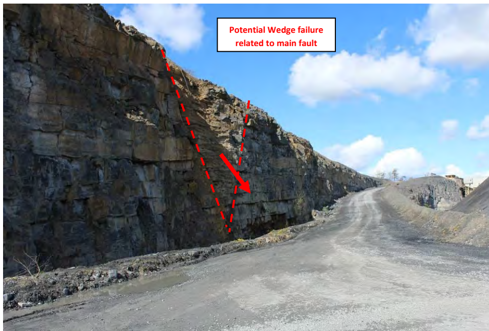
Figure 30 Potential Wedge failure related to main fault
