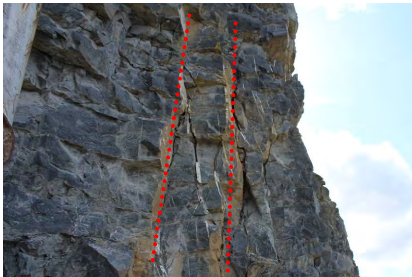
Figure 6 The secondary joint set (highlighted in red)
