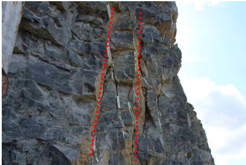
Figure 6 The secondary joint set (highlighted in red taken in 2020)
